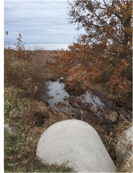
Main Channel at Garrison Oak Technical Park
